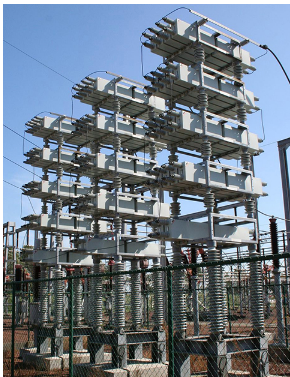
Figure 15.4.4: Power capacitors are used to balance the impedance of the effective inductance in transmission lines.
