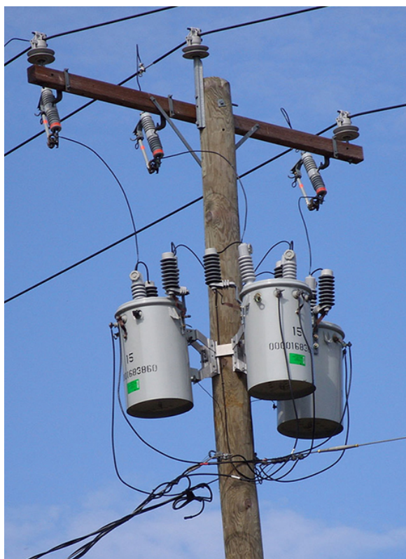
Figure 15.7.2: Transformers are used to step down the high voltages in transmission lines to the 110 to 220 V used in homes. (credit: modification of work by “Fortyseven”/Flickr)
