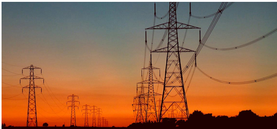
Figure 15.1.1: The current we draw into our houses is an alternating current (ac). Power lines transmit ac to our neighborhoods, where local power stations and transformers distribute it to our homes. In this chapter, we discuss how a transformer works and how it allows us to transmit power at very high voltages and minimal heating losses across the lines.
